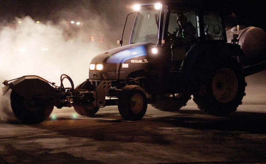
An airfield damage repair team clears debris during an operational readiness inspection at Kunsan. In addition to patching craters, such teams repair lighting and carry out myriad other tasks necessary to get the runway usable.
